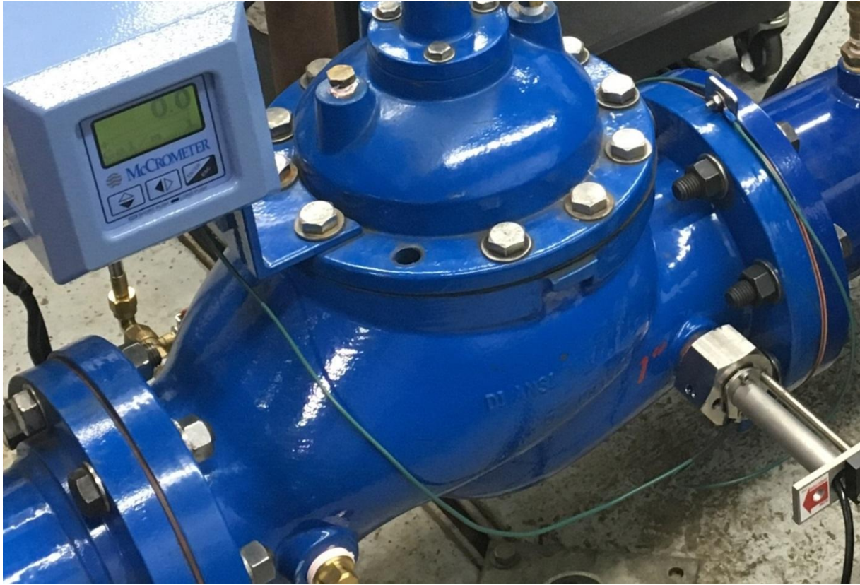
Figure 33: Converter & probe with ground wiring
